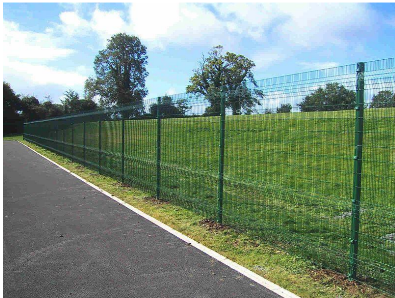
Fig 72. Illustrative example of 2.4m high paladin security fence
